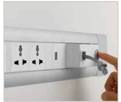
Flush mounting power & data module
